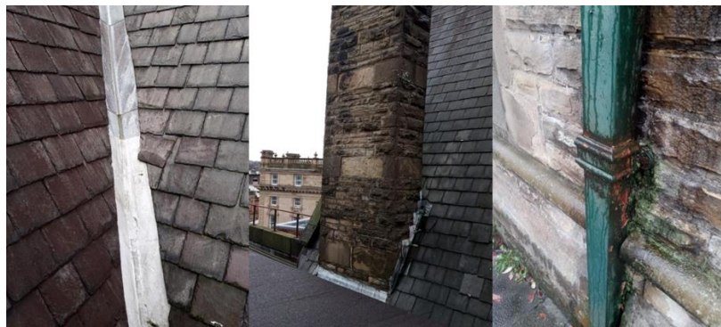
Figure Four – Photos of building defects
