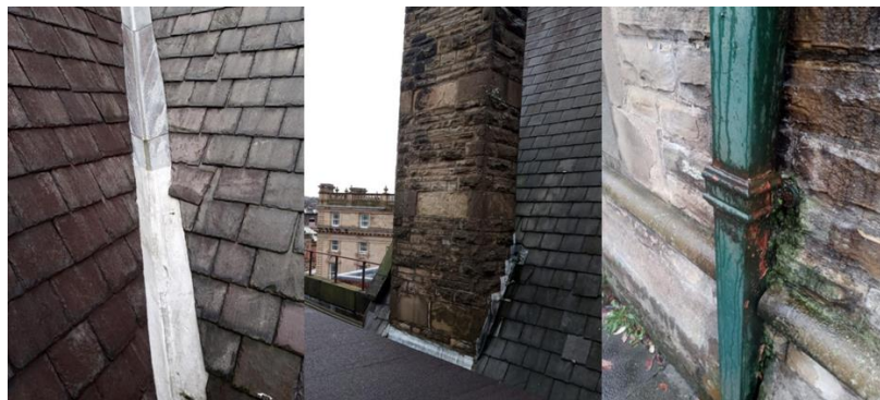
Figure Four – Photos of building defects
